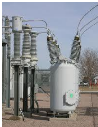
Figure 2. Voltage regulator monitors breaker status.
