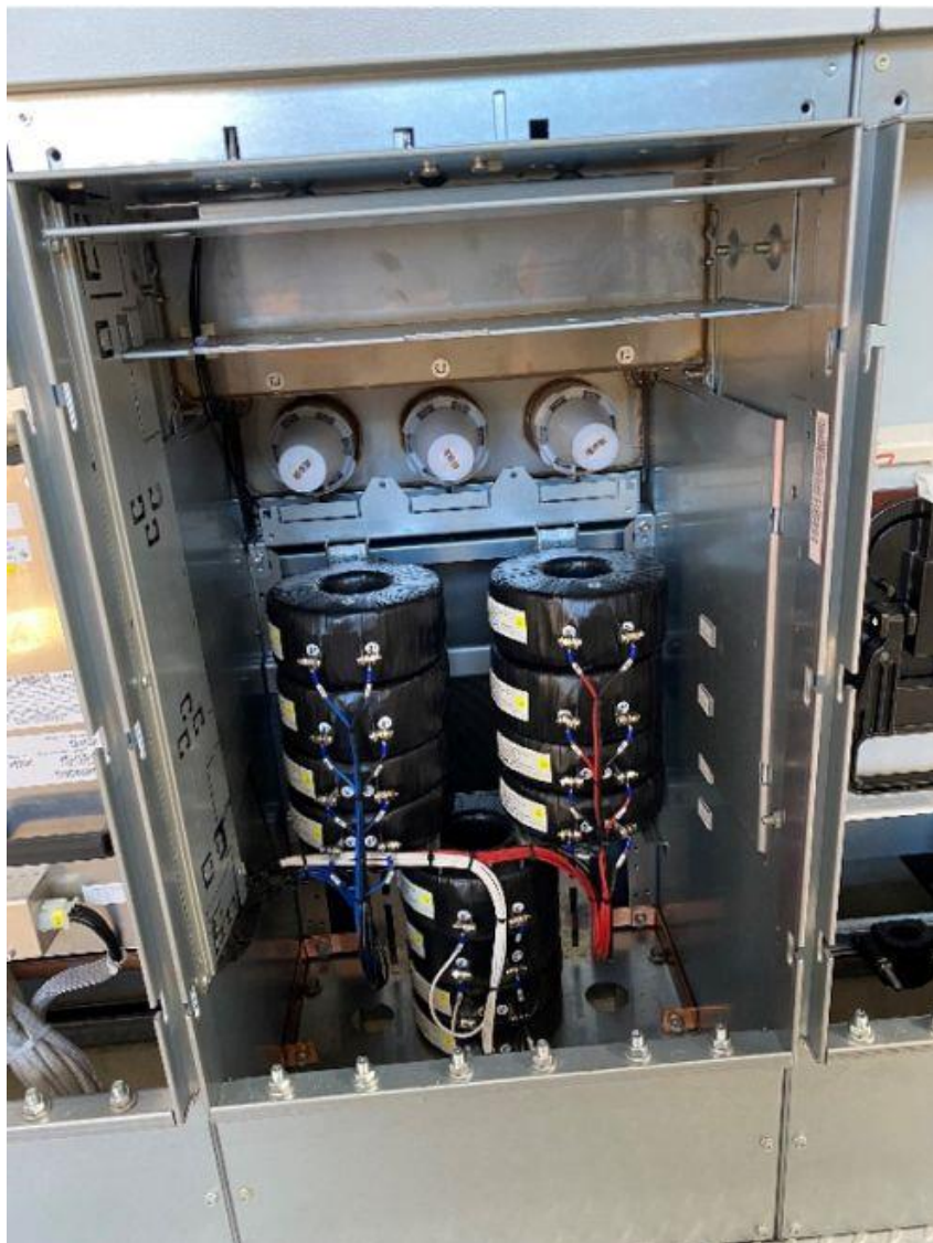
Figure 1. Four CTs in 8DJH cable compartment
